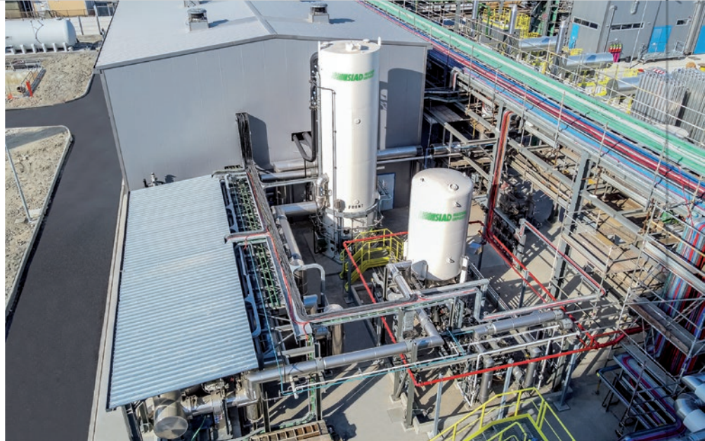
SMART TB-LNG BOG re-liquefaction plant Courtesy of DIG (Depositi Italiani GNL - Italian Coastal LNG Deposits), Ravenna, Italy
