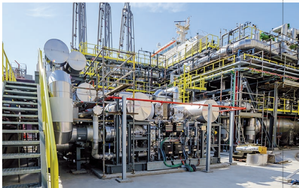
BOG compressors - Courtesy of DIG (Depositi Italiani GNL - Italian Coastal LNG Deposits), Ravenna, Italy
